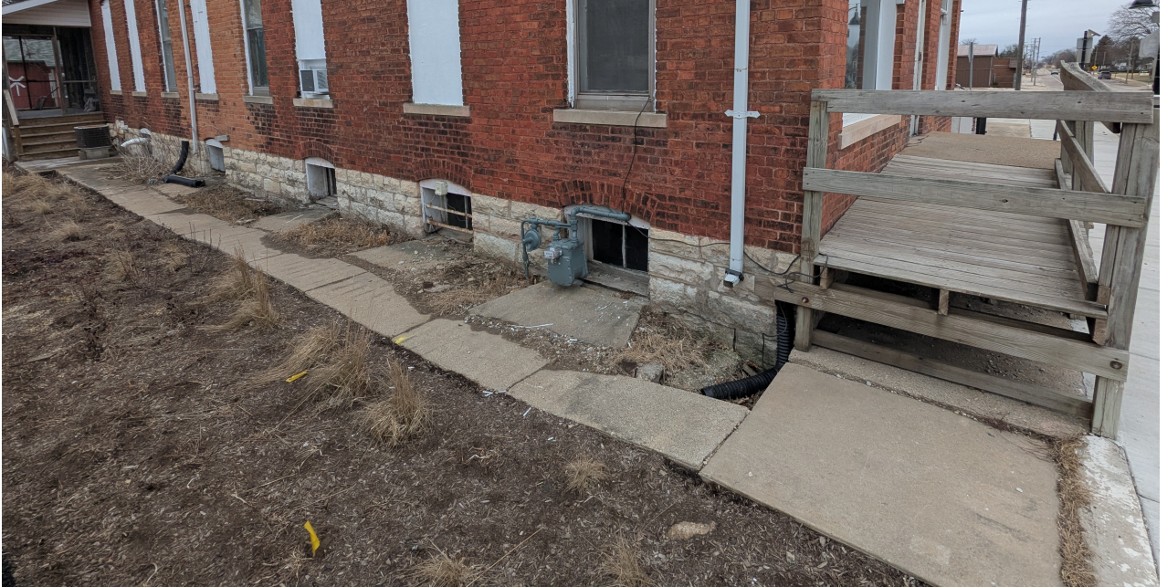
The “improvements” the handicap ramp was “in the way of”
